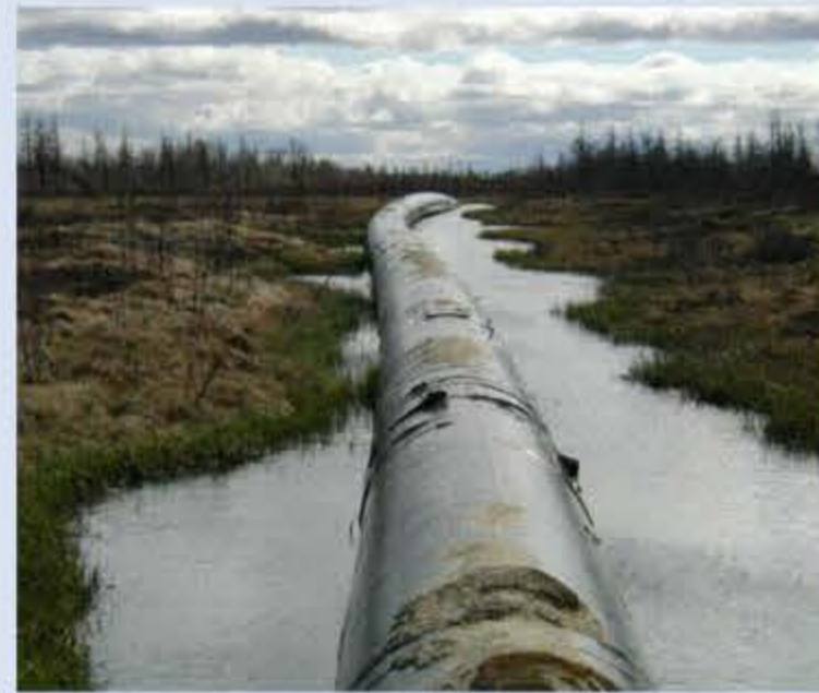
Upheaval of buried Urengoi-Center pipeline in western Siberia. (Brouchkov et al., Pipelines on Russian North: review of problems of interaction with permafrost)
